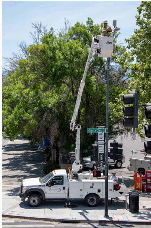
Field install of V5000 DN mounted at a downtown intersection.
