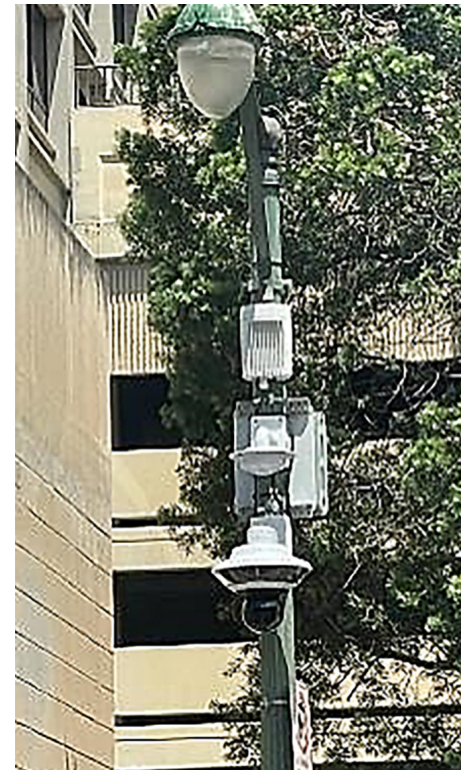
V5000 installation on city-owned infrastructure.
