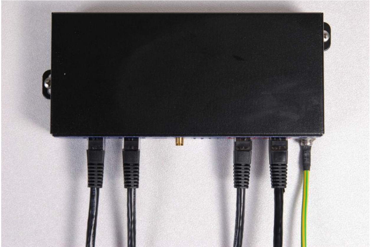
Figure 111 PTP-SYNC mounted on a wall
