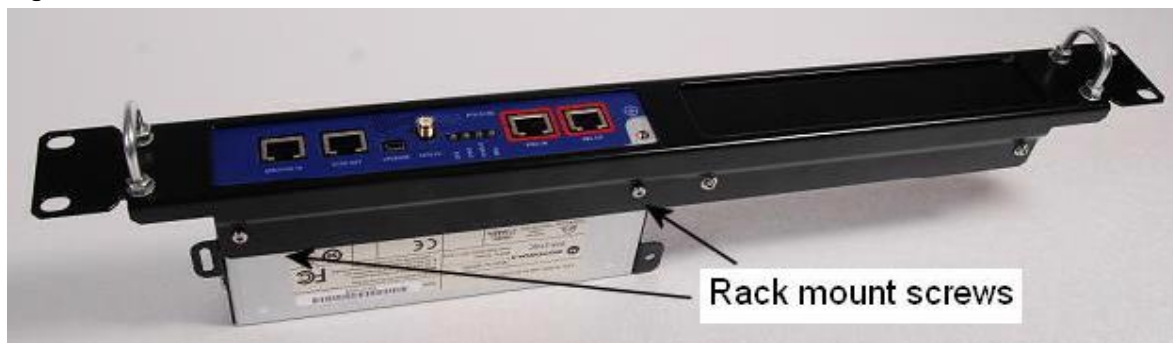
Figure 110 PTP-SYNC mounted in a rack
