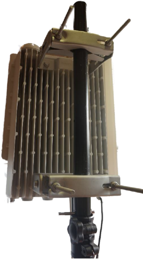
Figure 88: ODU mounted on the Mast
