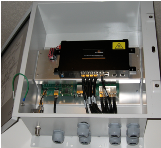
Figure 57: CMM4 (Cabinet with switch)
